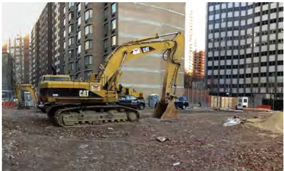
The site of the future College of Nursing building: Construction has begun on First Avenue between East 25th and 26th Streets!
