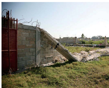
A wall of the FSIL nursing college in Haiti was destroyed in the earthquake.
